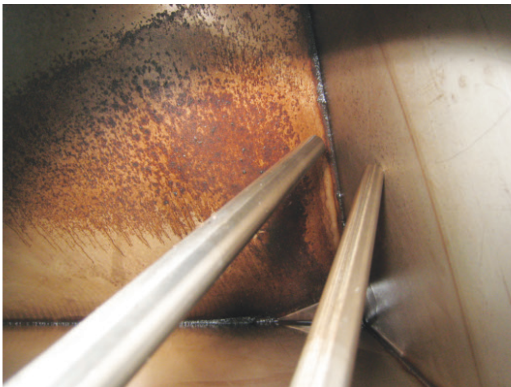
A pump may be able to get out the worst of the sludge, above, but you will still need to wipe down the tank. A weld/seam inspection, right, is an important step. Mmmm...sludge, opposite right
